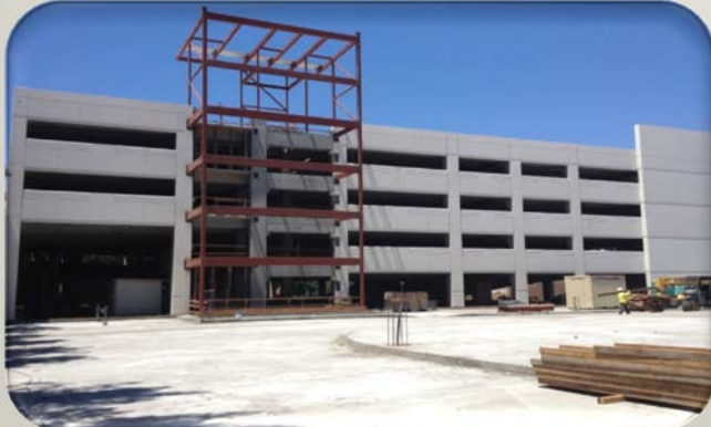
West elevation, large cladding panels on right. Steel stair tower in center.
