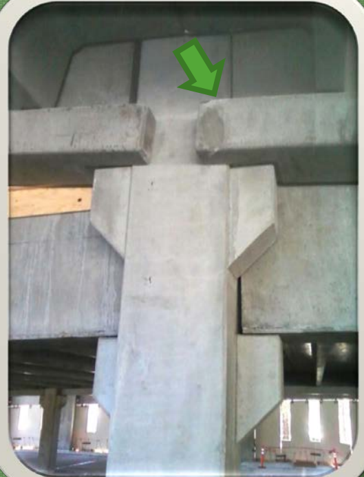
Lower LB tieback at interior, ledge projects from end of beam to resist torsional moment.
